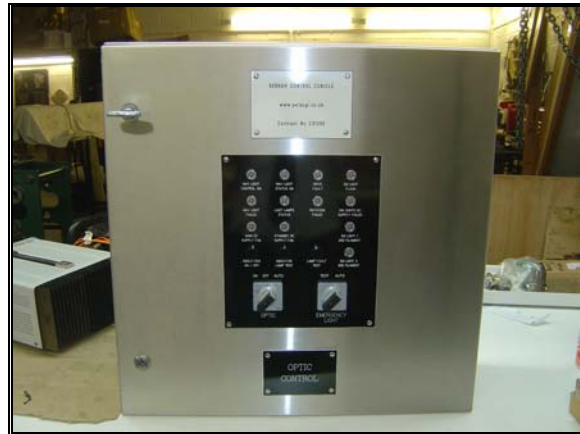
Earagh Central Control Cubicle
