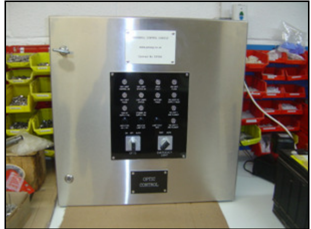
Rockabill Central Control Cubicle
