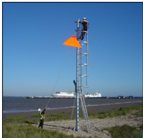
Assembly of day marks on to the 8 metre front tower showing Berths 3 and 4 behind.
