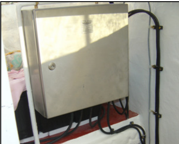
Telemetry power supply.
